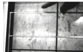
Fig. 10b: This crack has no effect on energy production.
